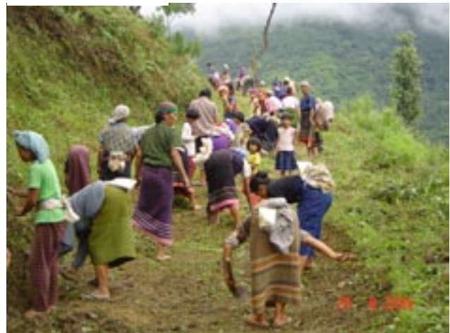
Local community at Khonoma clearing the path for a road- Khonoma Green villaae Project, Nagaland
