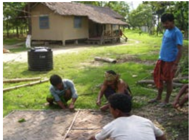
Building of cottages at the Manas Maozigendri Jungle Camp, Assam. The camp is run by the local community
