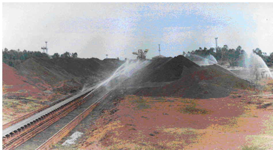
Fig. No. 5.2.3.1.5.1 Stockpile Water Sprinkling System
