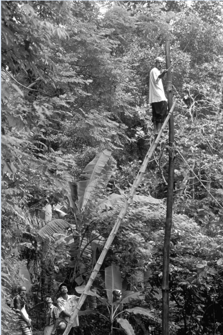
Villagers extending cables to provide village with electricity from hydro power. (Photo from the World Bank Photo Library.)
