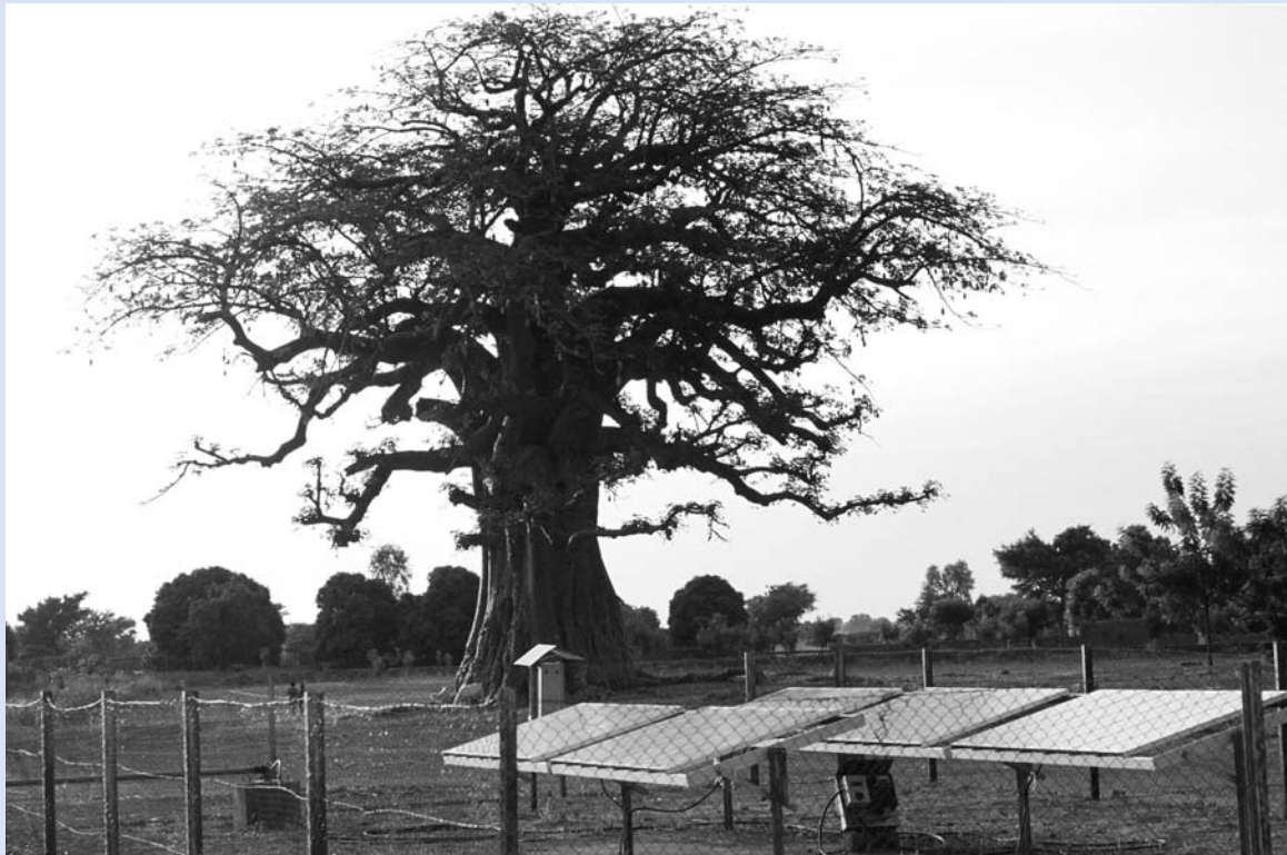
Solar panels in Mali provide rural power. (Photo from the World Bank Photo Library.)
