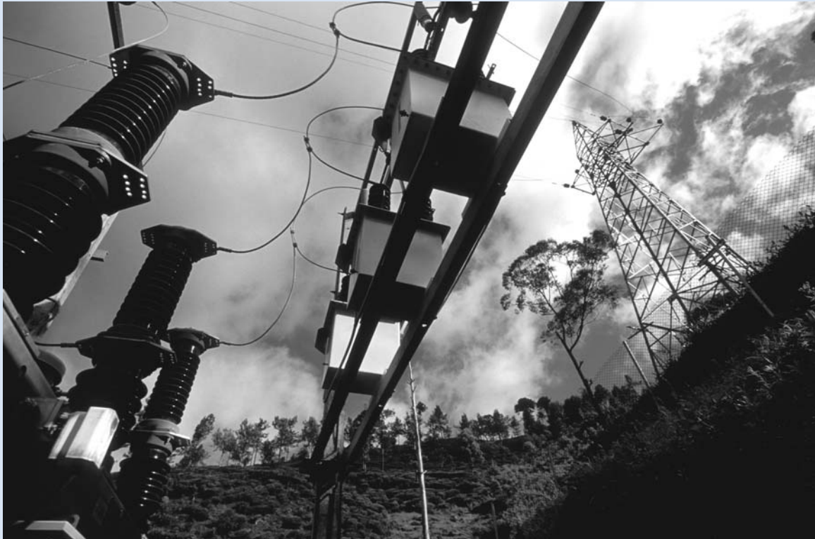
Electricity distributors at a mini hydroelectric plant in Sri Lanka. (Photo from the World Bank Photo Library.)
