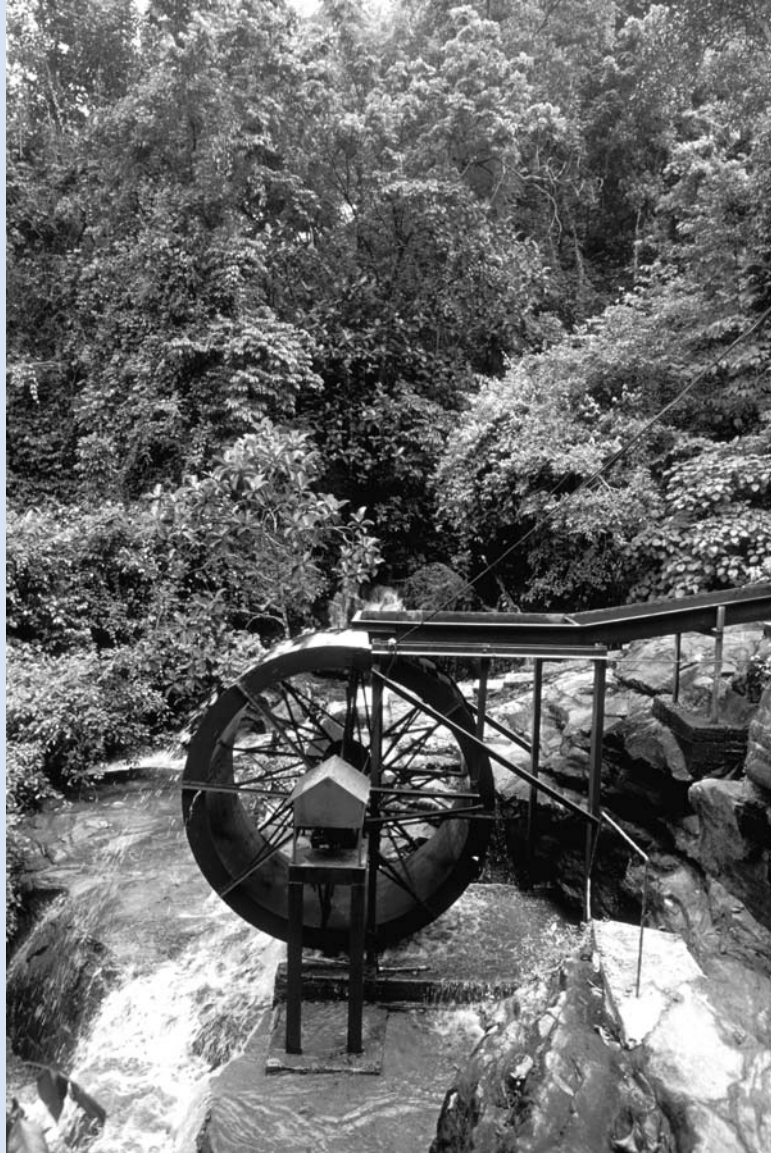
Turbine on stream near village generating energy as part of hydro scheme. (Photo from the World Bank Photo Library.)
