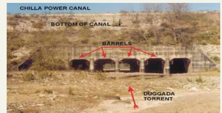
Figure 9 – Barrels of Duggada drainage crossing on the Chilla Hydro Power Canal in Rajaji National Park, Uttarakhand
