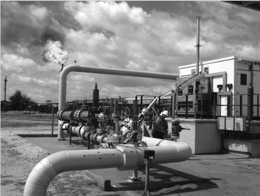
Gas flaring and pipeline equipment, SASOL Pipeline, Sub-Saharan Africa. Photo courtesy of SASOL/IFC.
