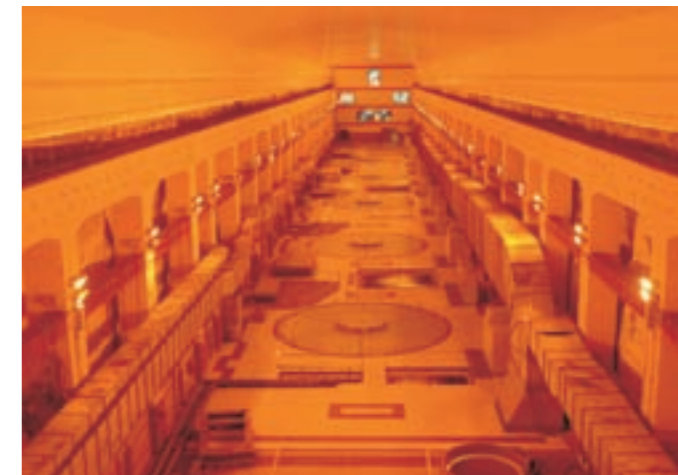
A view of Nathpa Jakhri Hydro Electric Power Station, Himachal Pradesh
