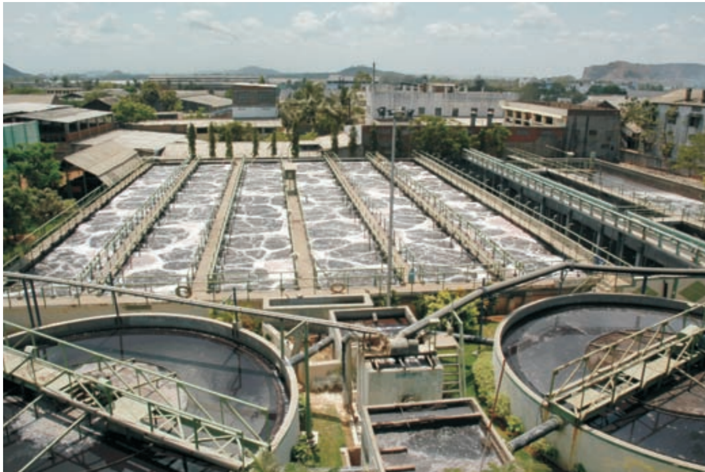
A common effluent treatment plant at Chennai
