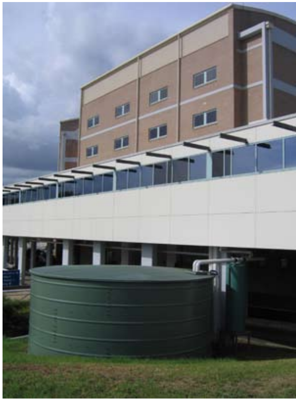
Rainwater Harvesting tank at hospital, Australia
