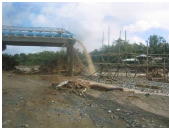
Flood-damaged main pipe for potable water for the City of Iloilo. Kahublagan
