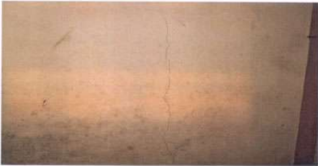
(Minor cracks shown to the committee by villagers in their houses)
