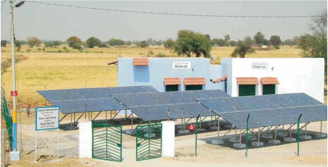
Community power plant at Rampura
