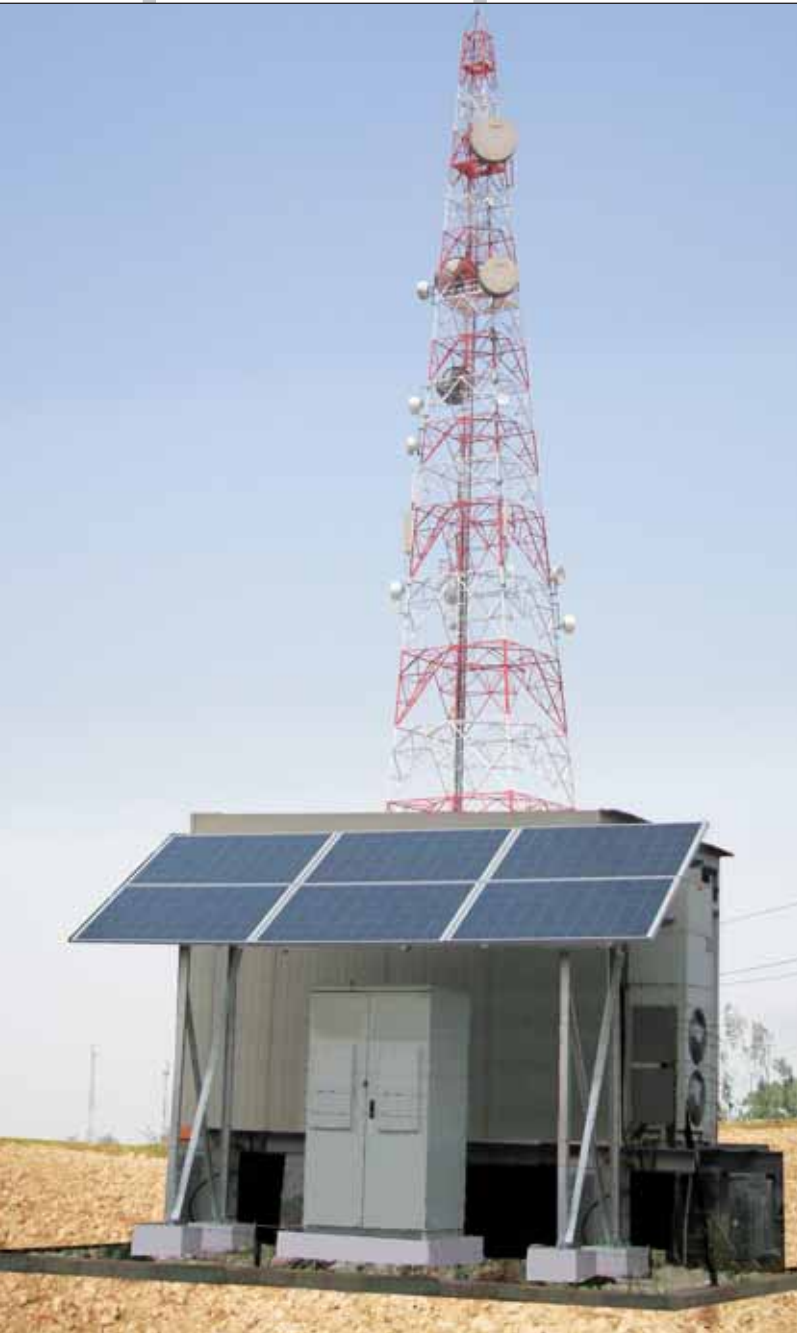
A telecom tower running on solar power
