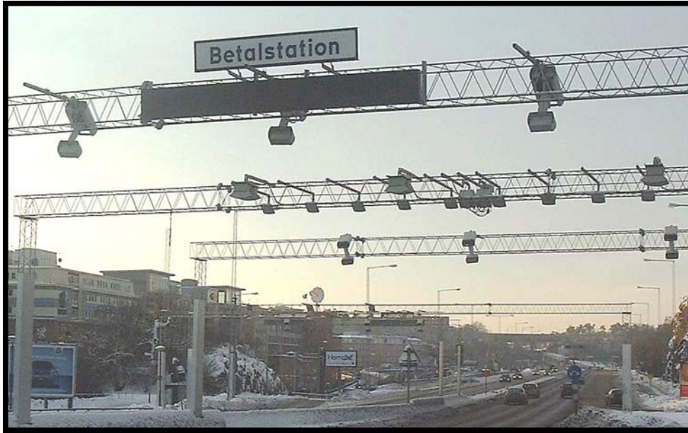
Figure 5: Stockholm congestion charging station (Source: Mats Halldin)
