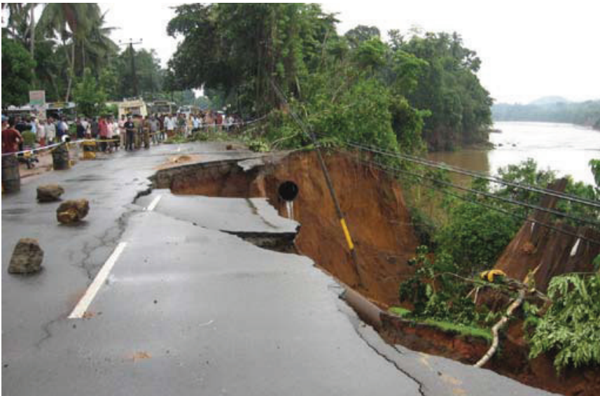
Figure 1. Kelani river bank erosion due to sand mining. A domestic water supply pipe line underneath the road got damaged and city water supply got disturbed for several days. (Photo: Badra Kamaladasa, Irrigation Department of Sri Lanka).
