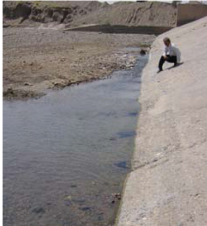
Figure 3. Water emerging from weepholes
