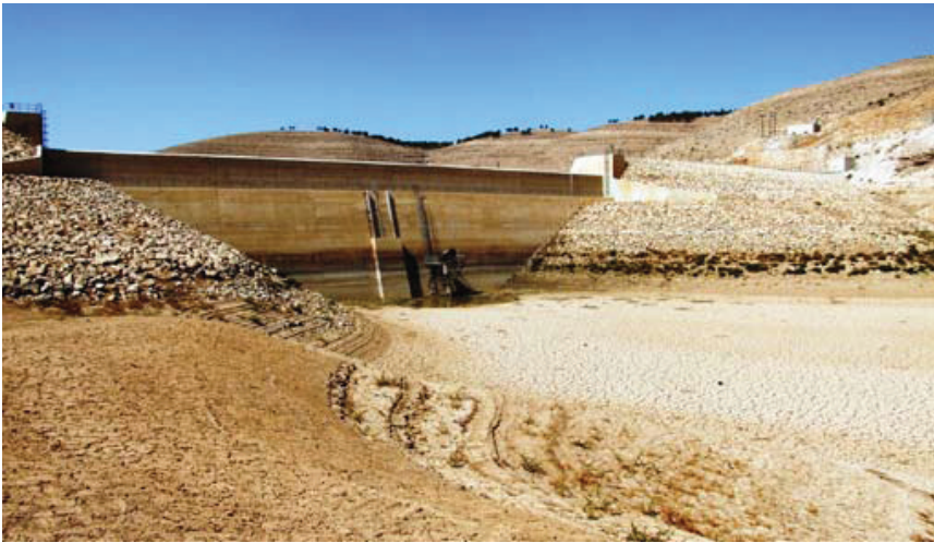
Figure 3: Sediment Accumulation at the Bottom of the Wadi Wala dam has led to the Closure of the Bottom Outlet and the lower Draw-off Pipe
